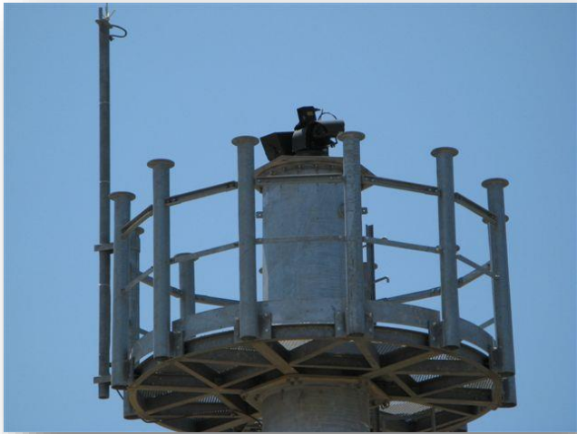
Figure 7: Close-up of tower mount.
